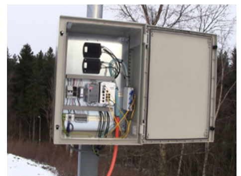
The live footage from the thermal imaging cameras is encoded and transported to the control station through fiber optic cables.
